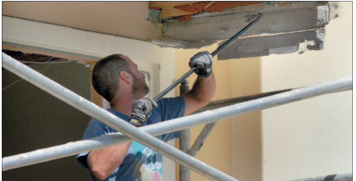
WATER DAMAGE: Between 22,000 and 89,000 homes are, or could be, leaking.
